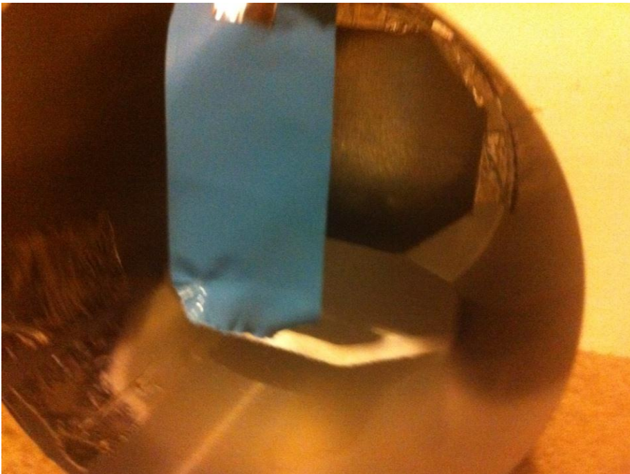
Figure 14: Thermal Battery Air Outlet
