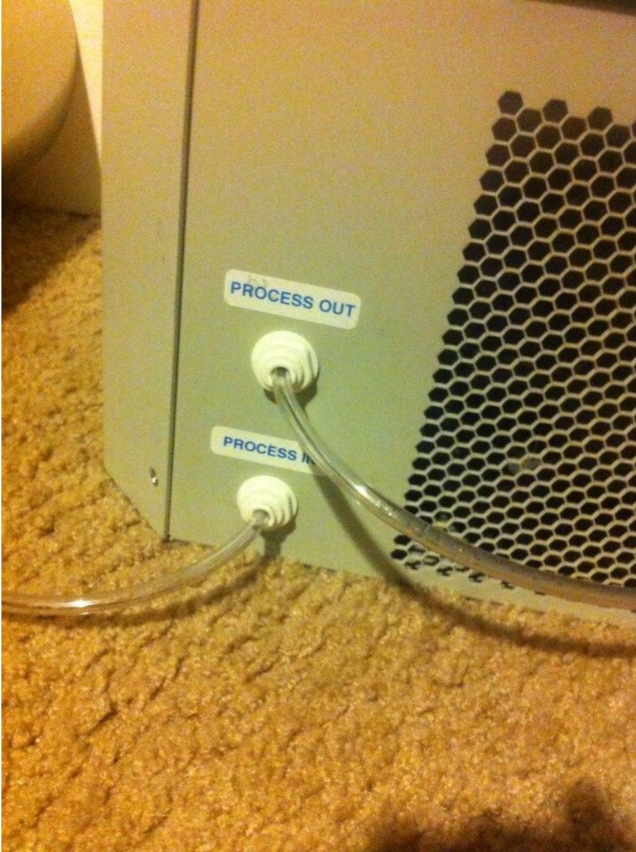
Figure 12: Chiller Process Tube Connections
